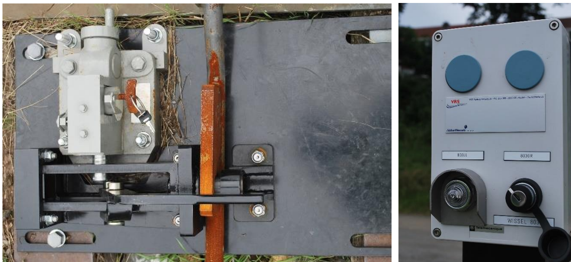
Figure 8. Left: manual operated point with mechanical lock, Right: electronic key box for remote controlled point
